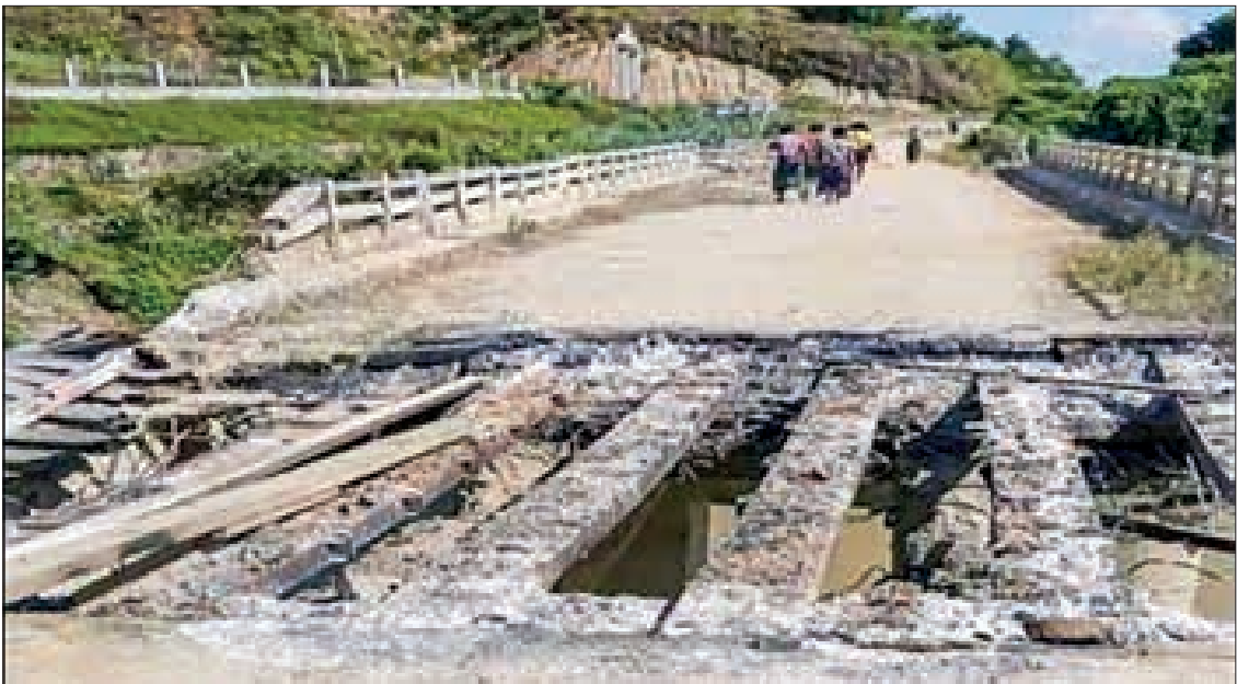
This image shows the Paluzawa Bridge on the Kalay-Mawlaik Road destroyed by PDF arson attack.
