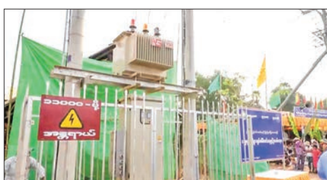
This photo showcases a substation facility that supplies electricity to a village in Magway Township.
