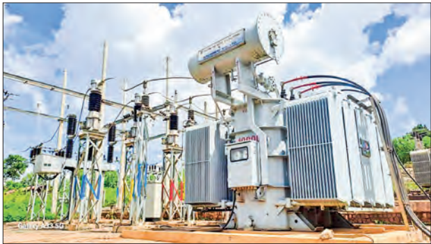
This image shows the transformer at the Kyaukme (Panpaung) Substation in Kyaukme.
