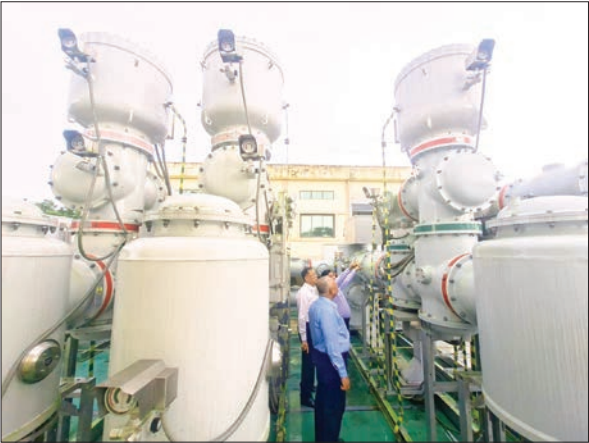
Deputy Minister U Aye Kyaw inspects transmission and distribution of electricity from a substation in Yangon yesterday.
