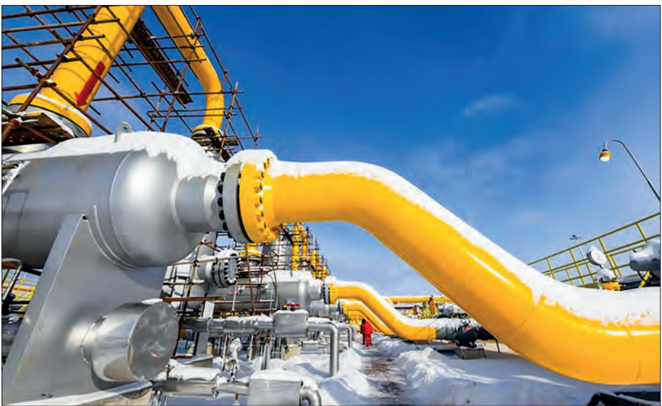
Photo taken on 19 November 2019 shows the China-Russia east-route natural gas pipeline in northeast China's Heilongjiang Province. PHOTO: XINHUA/FILE
