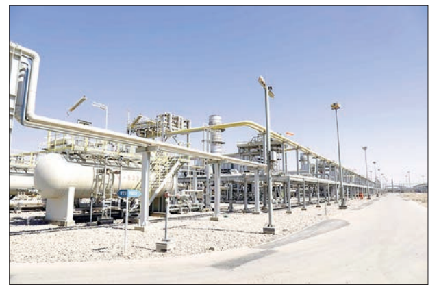
Photo shows a power plant in Halfaya oil field in the southern Iraqi province of Maysan on 25 September 2022. PHOTO: XINHUA/FILE
