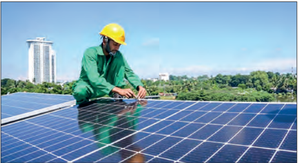
Sri Lanka aims at expanding rooftop solar generation. PHOTO: ADB/FILE
