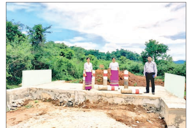
Officials oversee the completion of the production road culvert project in Mongshu.
