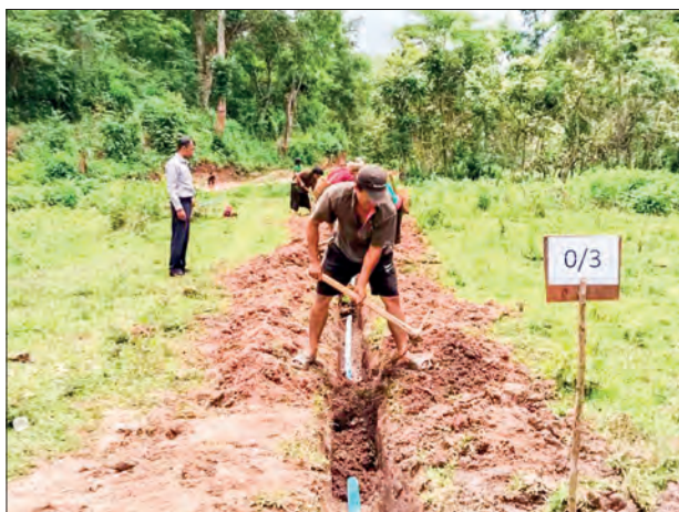
Inspection of the rural water supply project is in progress yesterday in Kunhing Township, southern Shan State.
