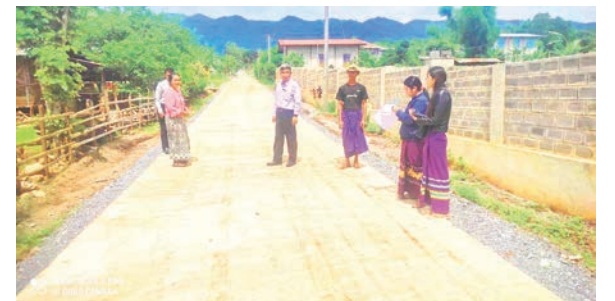
Officials oversee the ongoing construction of a village entrance concrete road in Taunggyi Township, southern Shan State.
