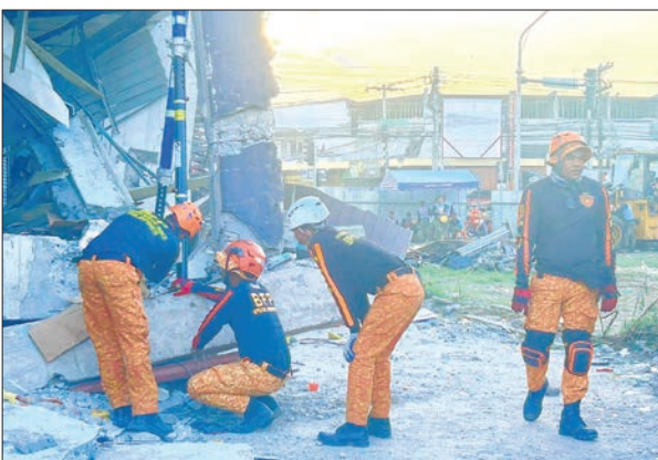
Responders conduct a rescue operation at a collapsed building after a 7.8 magnitude earthquake in General Santos City on 8 June 2026. PHOTO: AFP
