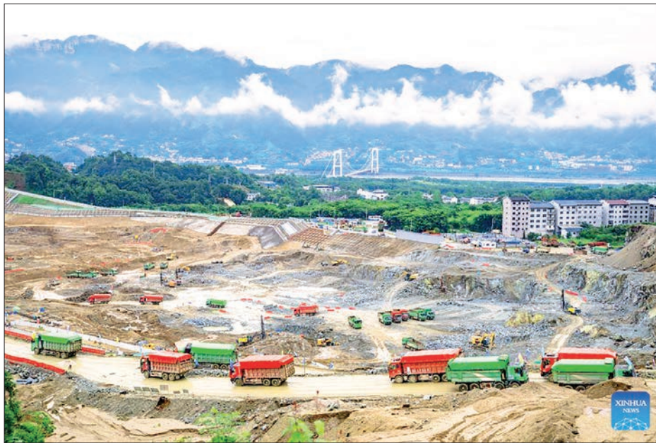
This photo taken on 8 June 2026 shows the construction site in an early-phase excavation zone of the Three Gorges new waterway project in Yichang, central China's Hubei Province. PHOTO: XINHUA
