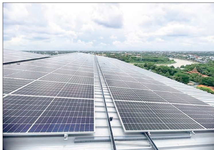
An array of solar panels generates renewable energy.
