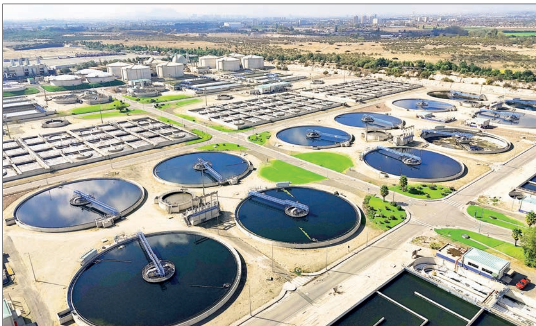
Aerial view of a wastewater treatment plant, known as biofactories, where the waters of the Mapocho River are treated in Santiago on 7 May 2026. PHOTO: FRANCO FAFASULI / AFP
