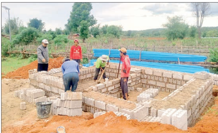
This image depicts the ongoing implementation of the Kehsi Rural Water Supply Project.
