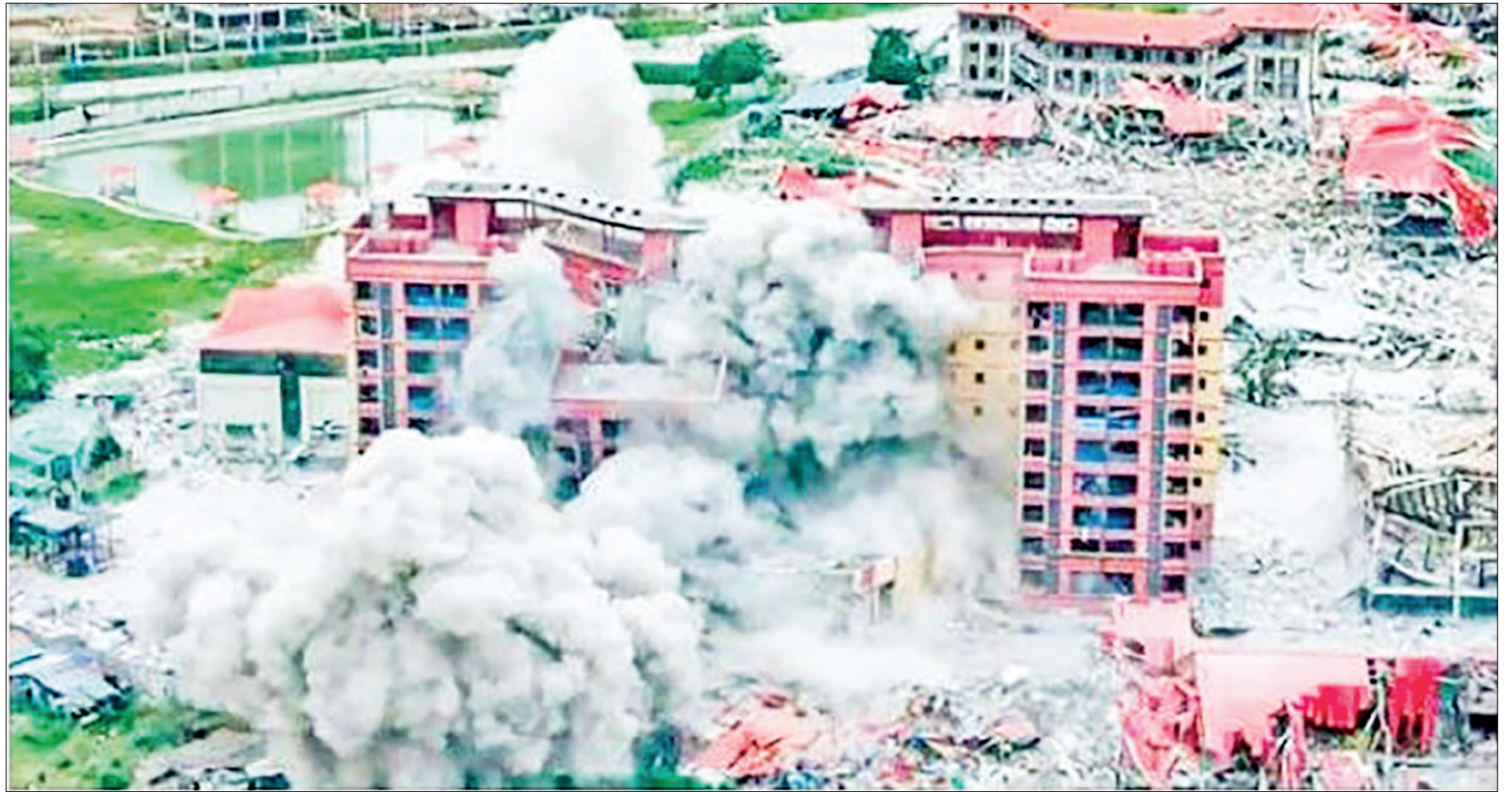
This photo shows the demolition of the building used to commit telecom fraud and online gambling in the KK Park area.
