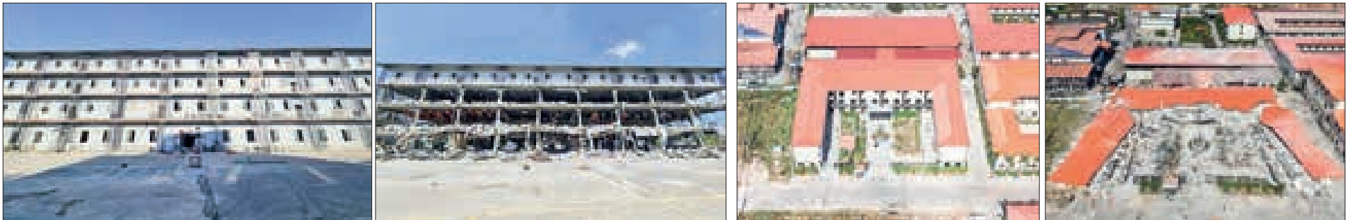
These four photos reveal the illegally built four-and two-storey flats before and after the demolition in the KK Park Section 3, Myawady Township, Kayin State.
