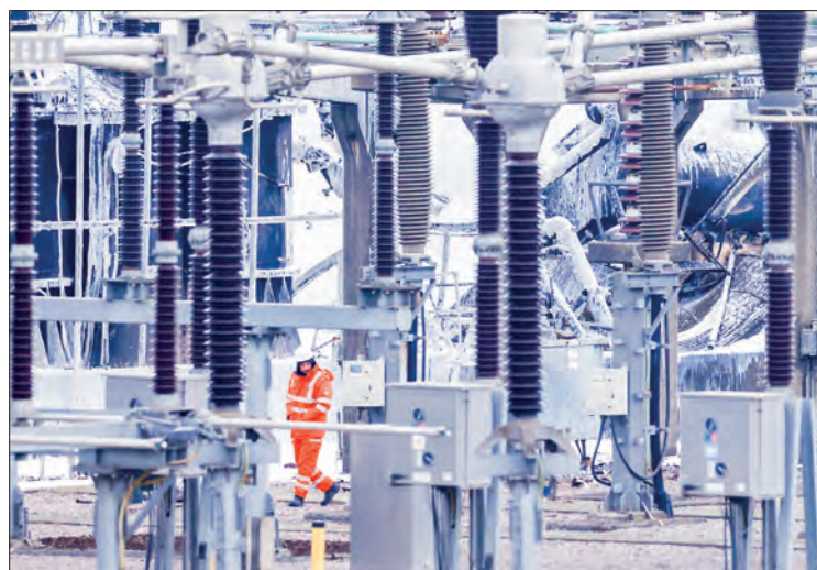
A staff member walks past a substation supplying power to Heathrow Airport where a fire broke out in Hayes, west London on 21 March 2025. PHOTO: AFP
