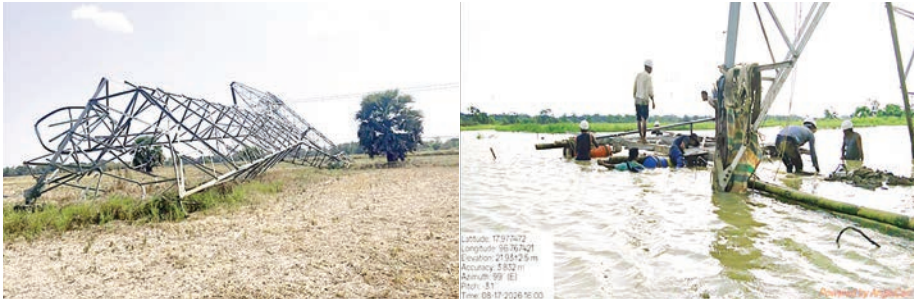
Images show a collapsed tower and MoEE employees repairing the damage.
