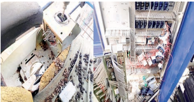
This image shows the damage to the control room of the tower crane.
