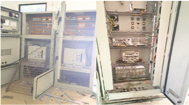
This photo reveals the destruction of the machine panels.
