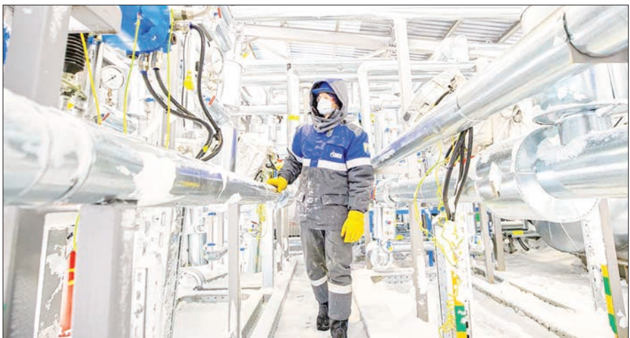
A worker inspecting complex insulated piping and industrial processing equipment at a Gazprom energy facility. PHOTO: GAZPROM
