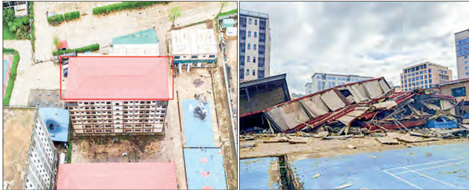
Images show the update before and after the demolition of the nine-storey scam hub.
