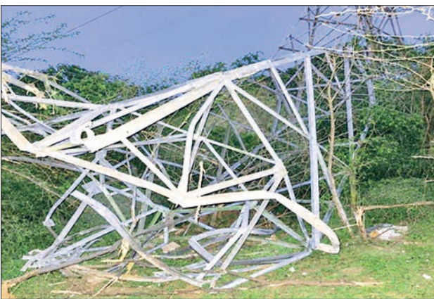
A power tower brought down by a blast perpetrated by terrorists.
