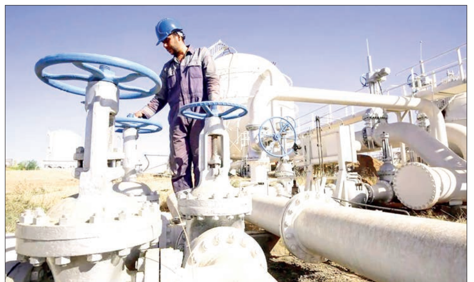
An Iraqi oil employee checks pipelines at the Bai Hassan oil field, west of the northern Iraqi city of Kirkuk. PHOTO: AFP/FILE
